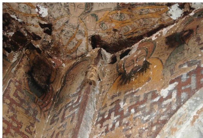
Fot. 10. Wukro. Visible manifestations of the destruction of 15th-century paintings covering the ceiling of Cherkos Church (photo by W. Florek 2011)
