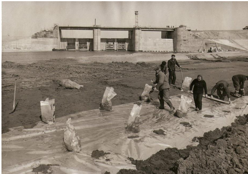
Fig. 2. Lining a part of the lake bottom with foil during its construction (photo by: A. Kobalczyk's archive)
